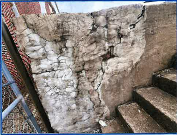
Evidence of wall movement after repair
