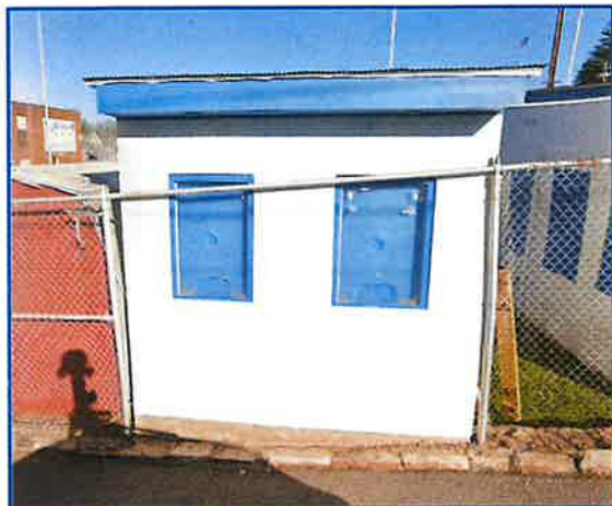
Tickets purchased from street side, top of wall may cause tripping hazard
