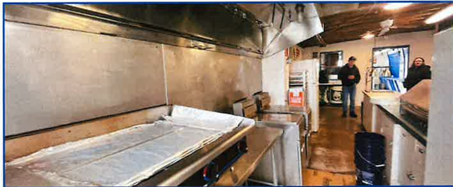
Exhaust hood over grille and fryers
