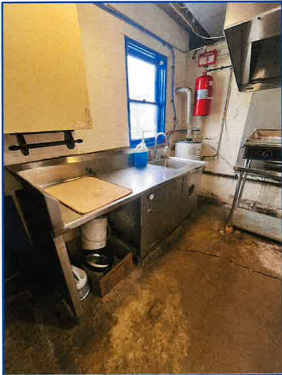
Floor is sinking/settling 3"-4" in back corner.
