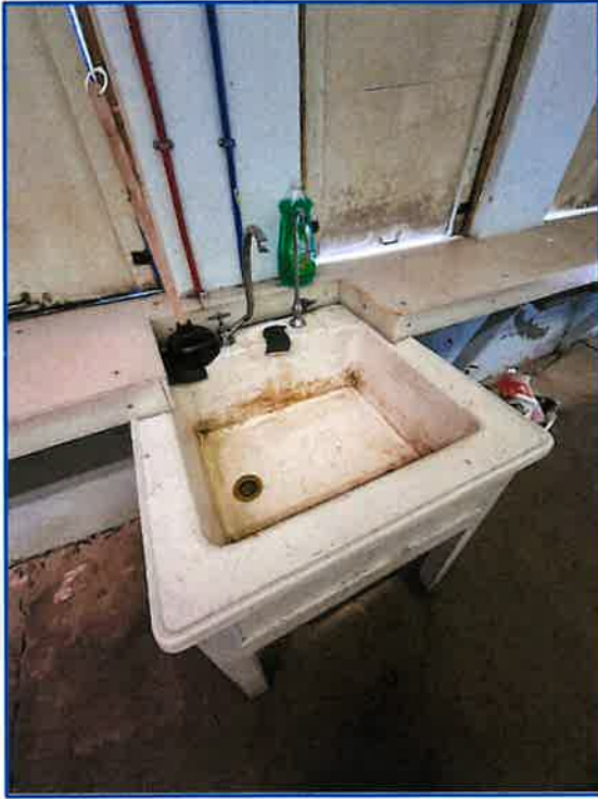
Inadequate dishwashing available
