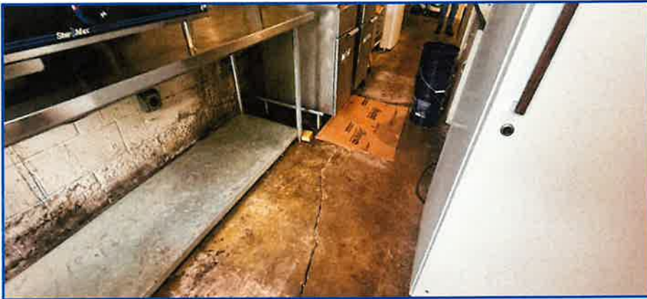
Grease or mold on wall below grille
