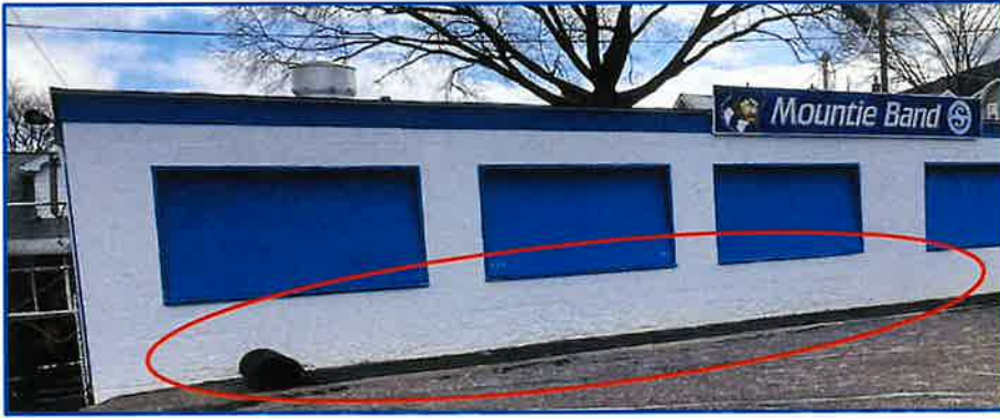
Water behind paint
