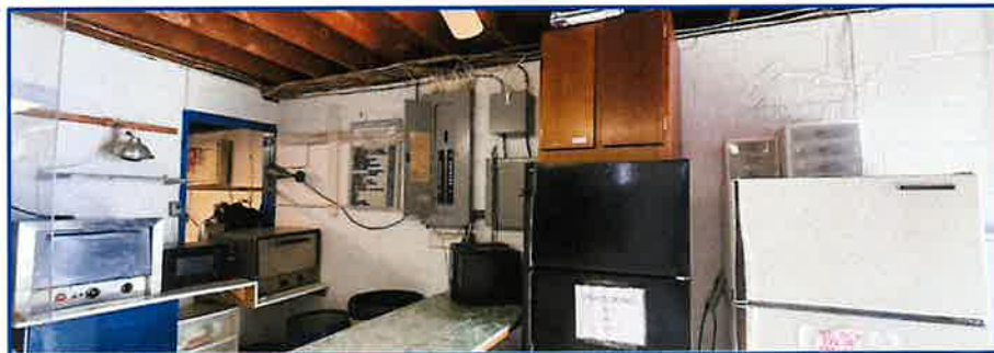
Electric panel close to capacity
